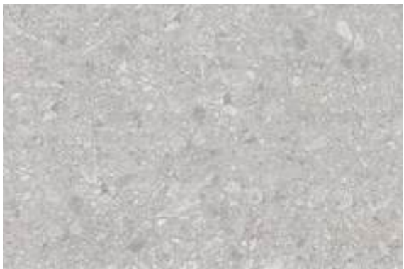
BATHROOM FLOOR & WALL
